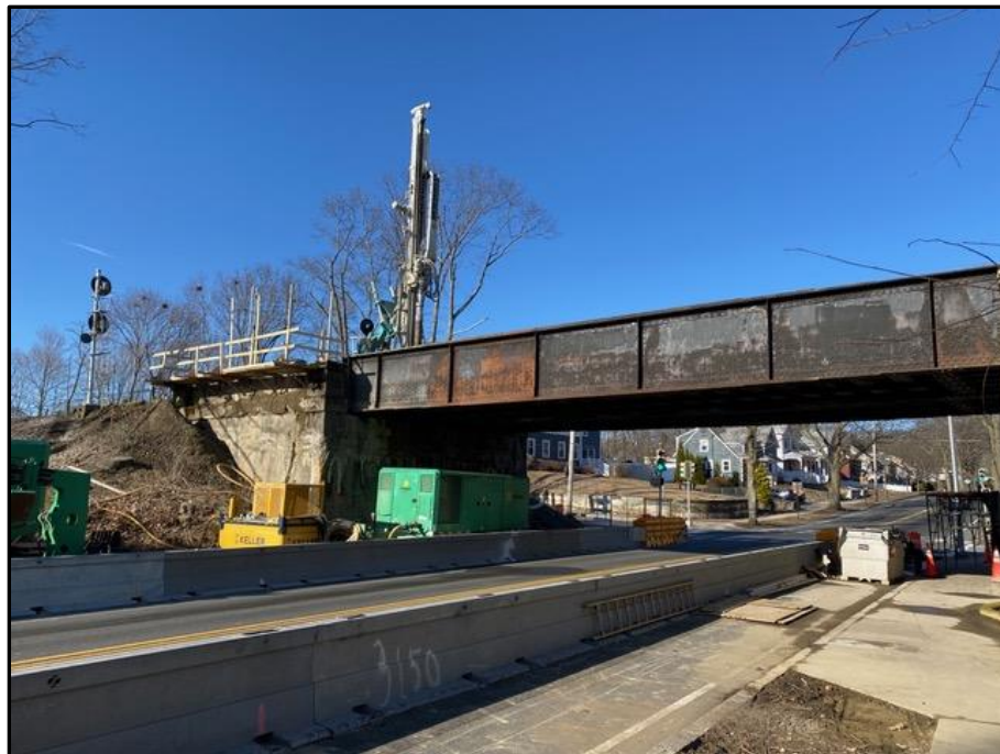
The 1929 steel bridge that carries the Western main line over Lynn Fells Parkway in Melrose will be replaced soon due to its age and current condition. This picture from April 3rd, 2021 shows the initial preparations being done to the bridge to get it ready to be removed. The new bridge will help provide more reliable service on the MBTA Commuter Rail line that uses it. Andrew Riedl photo.
