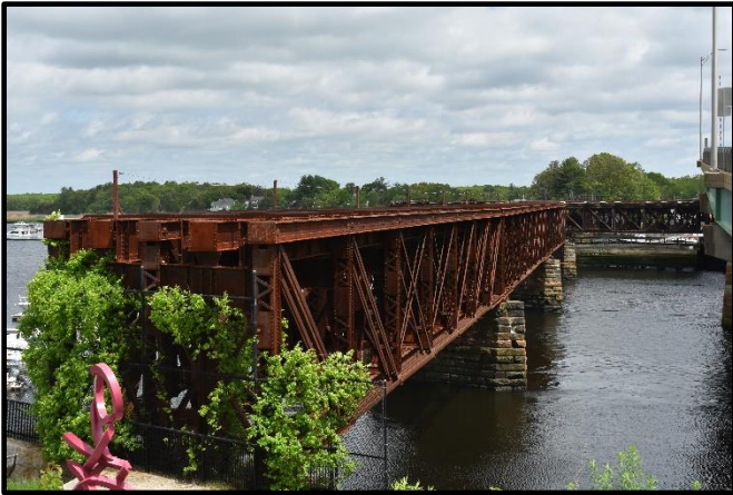
The massive iron swing bridge over the Merrimack River at the end of the Clipper City Rail Trail in Newburyport. Left in this open position since 1965, the open center swing span can be seen in the distance on the right, this cut the Eastern Route from a mainline between Boston and Portsmouth into two branch lines. The embankment leading up to the bridge has been demolished for trail construction.
