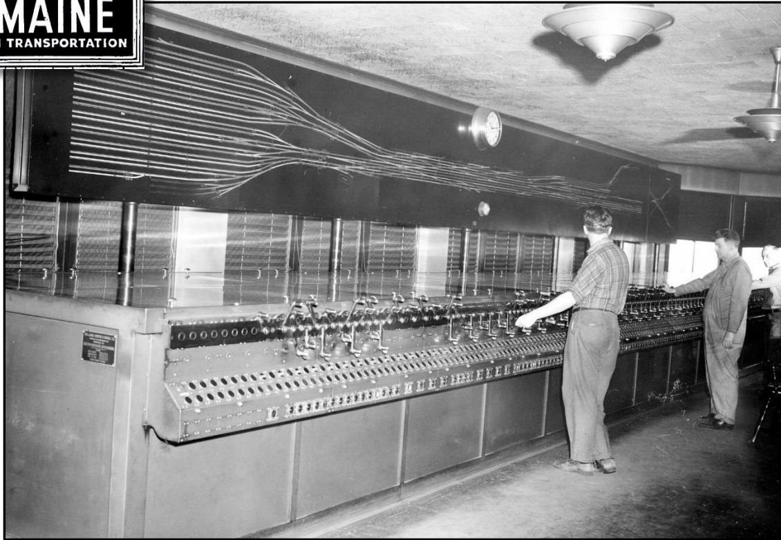
The control room at Tower A, Boston Terminal, as seen on March 5, 1947. Digital image made from photograph in Harry A. Frye Collection, B&MRRHS Archives. Cat. No. 2001.21.13.
