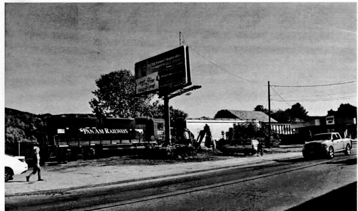
The very first train to traverse the Adams Branch extension between Cook Street and Hoosac Street in Adams is this Pan Am stone train seen dumping ballast along the track on October 3.
