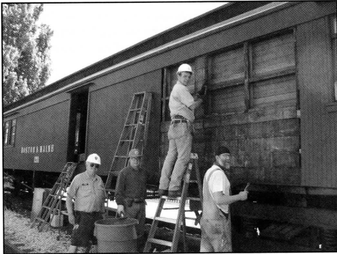
Dan Hyde, Dan Hovey, Jim Nizus and Bill Coffee pose for the camera while replacing siding on the combine.
