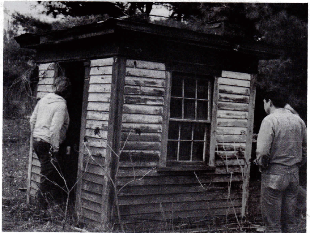
The B&MRRHS finally has its first B&M structure! This crossing shanty was formerly located in Exeter, NH, at either the Front Street or Main Street crossing. Though externally somewhat the worse for wear, it is structurally sound, and will be moved for restoration and final placement. Joe Shaw (in door) and Rob Quagan inspect the building recently. Restoration schedules will be published. See you there?
