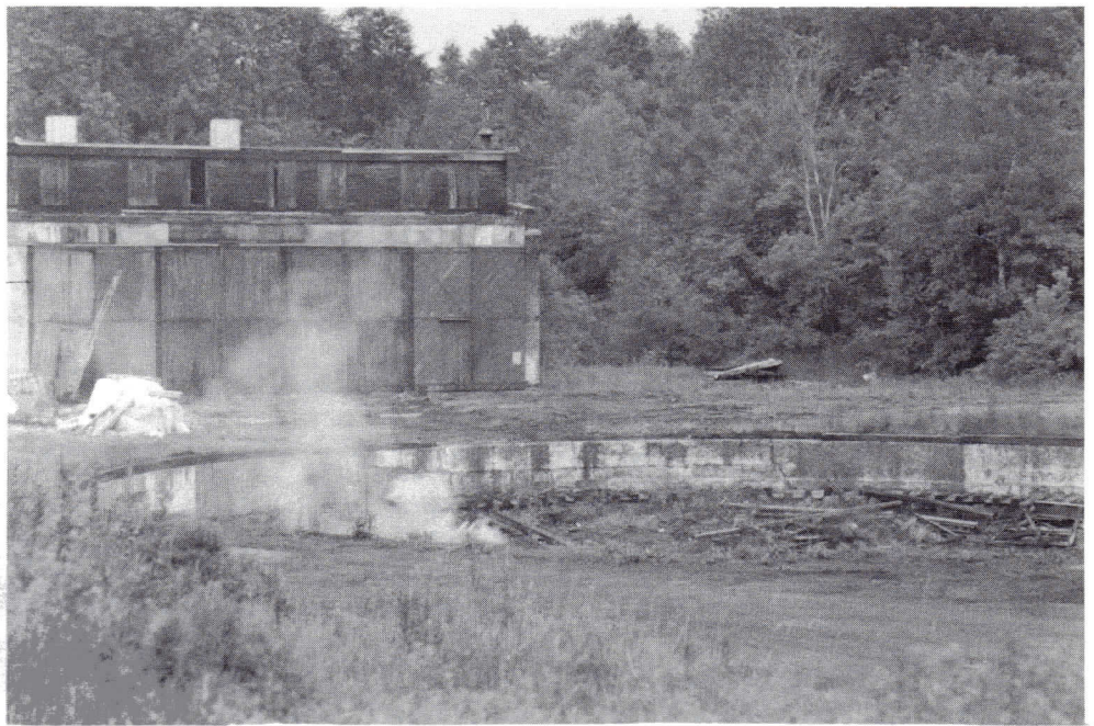
Demolition of Dover NH continues with the recent removal of the turntable bridge. The coachyard was also recently removed, and the tracks leading to the turntable were removed several years ago.
