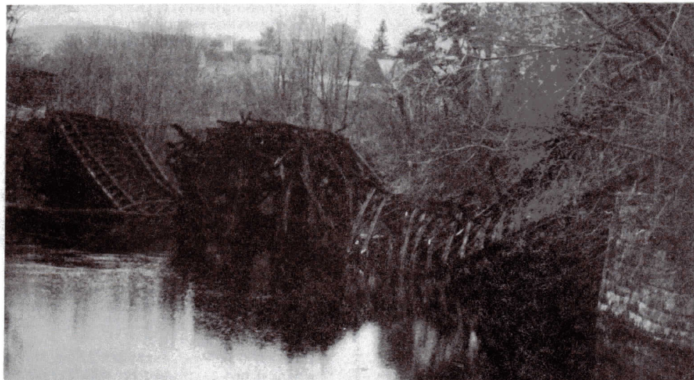
This photo illustrates the damage to the Hillsboro covered railroad bridge caused by arson (a Halloween prank). A 19 year old youth has been arrested and charged with arson. Photo by Harry Frye.
