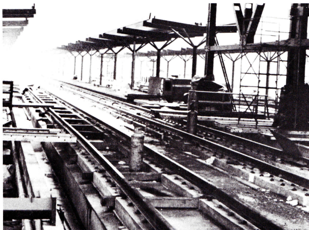
North Station reconstruction continues, with a target date for reopening of April 1985. Photo by Jeff Ursillo.
