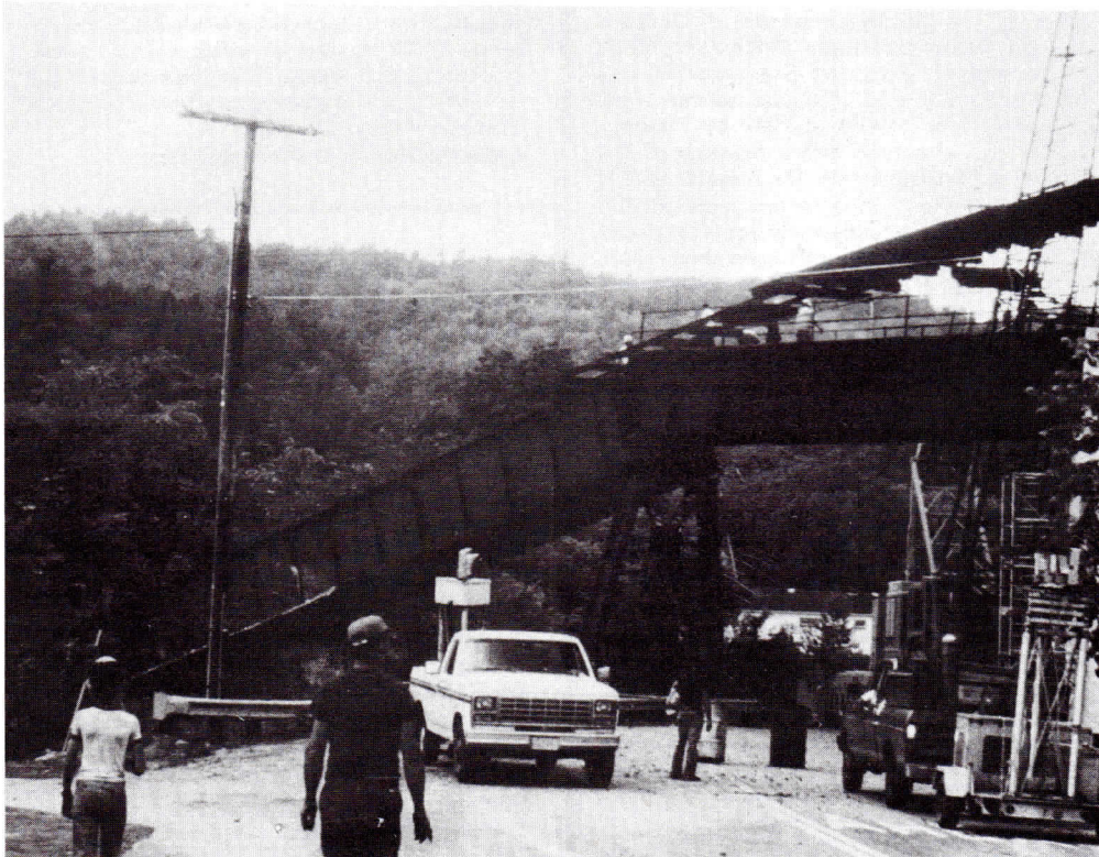
Extensive damage to the Wells River bridge is shown in this photo by Roger Robar. An undermined abutment (due to recent heavy rains) was the cause of the collapse.
