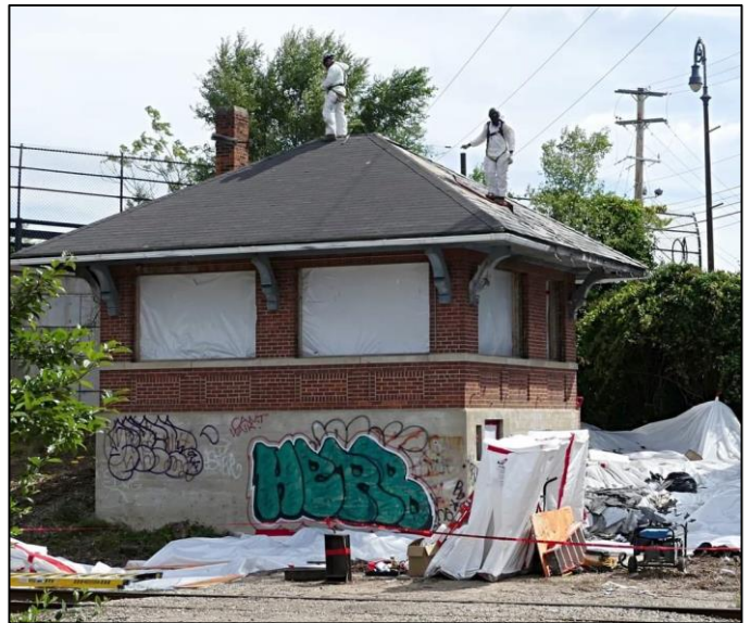
ABOVE: Concord Tower being prepped for demolition on August 9. Jesse Mazzie photo.
