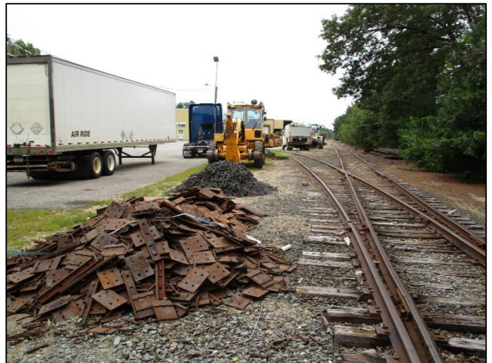
BELOW: Track equipment, ties, tie plates, and spikes staged near the airport in Nashua for rehabilitation of the Hillsboro Branch. Benjamin Campbell photos.
