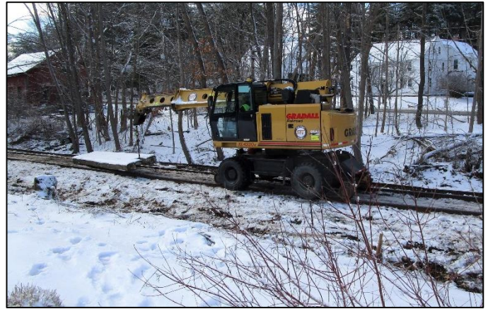
Bottom Left: Rails on the Central Mass Branch at Route 20, looking east before removal in March. The section house will be saved.
