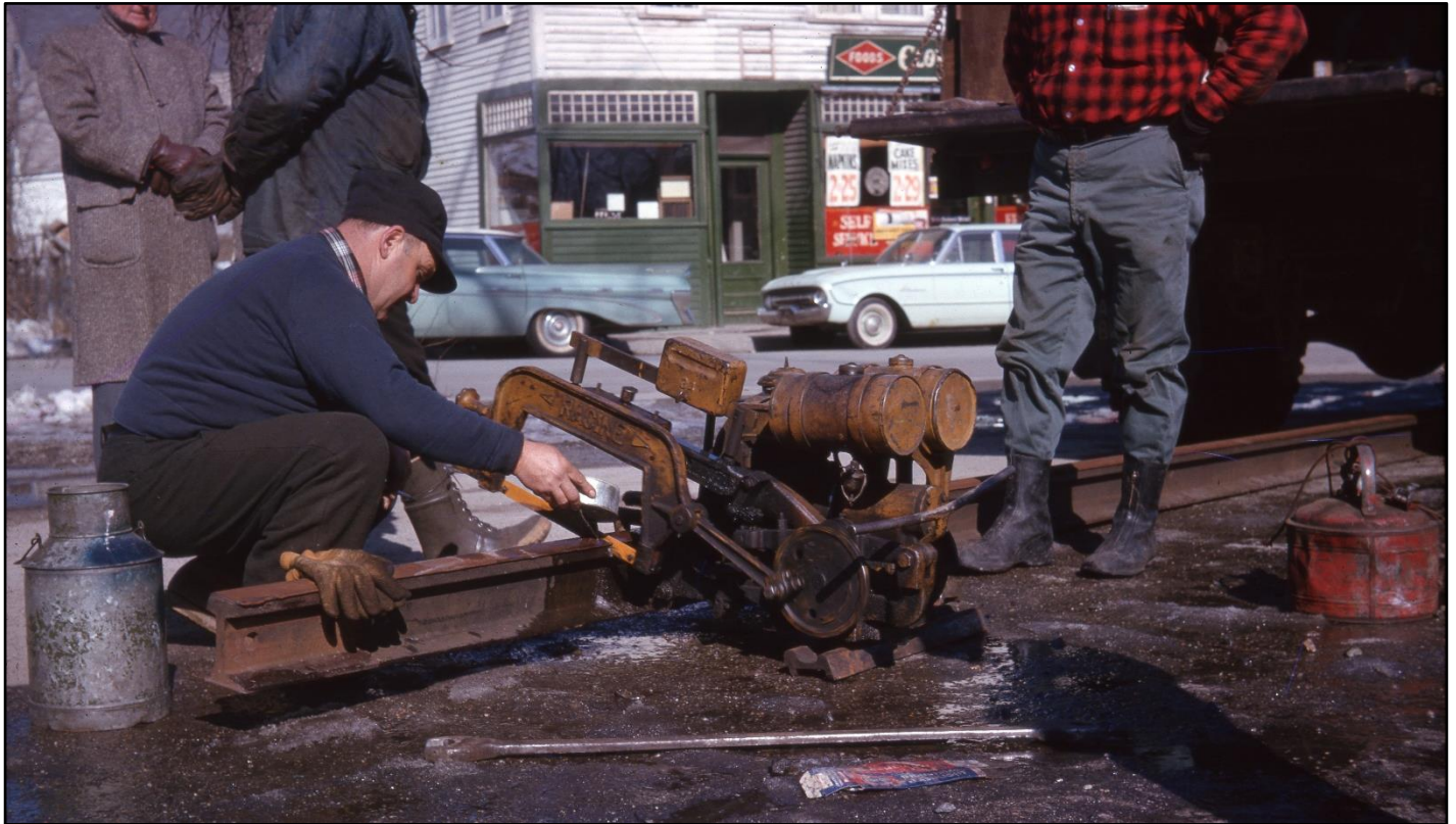
A worker cuts a length of rail during the clean-up of the wreck at Forge Village, MA on the Stony Brook Branch, 1964. These men, and their machines, no doubt got quite a bit of use in the 1960s and 1970s when it seemed that the B&M was having a major mishap nearly every week! H. Arnold Wilder photo, B&MRRHS Archives.
